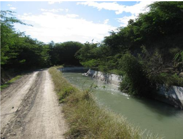
People that live along the highway get water from a trench diverted from this hydroelectric canal.
