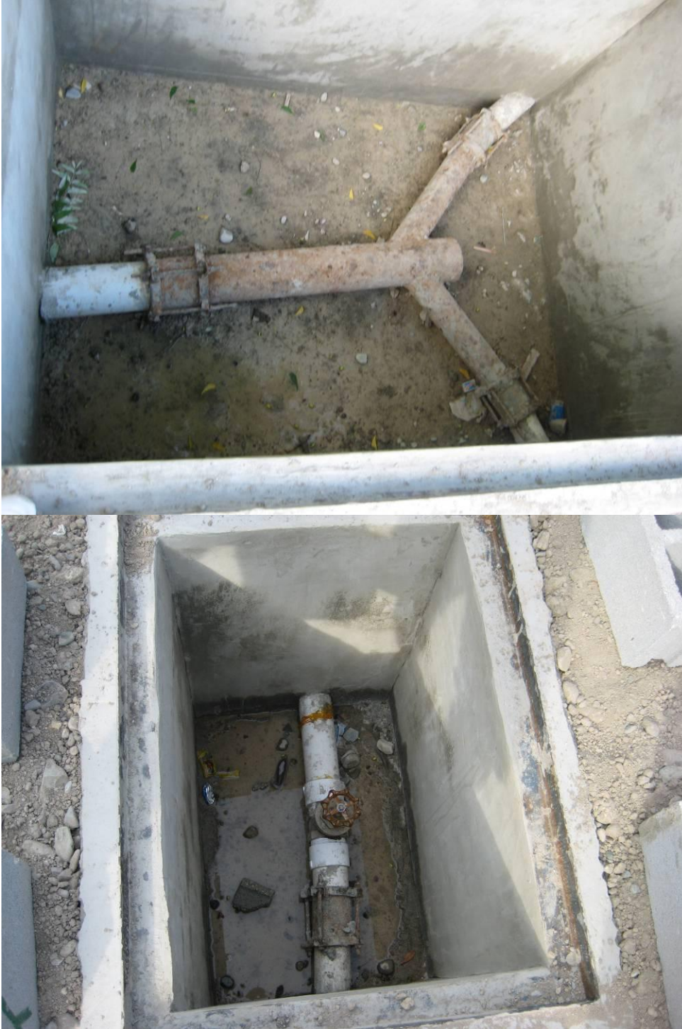
Figure 3-10: Distribution System Manholes
