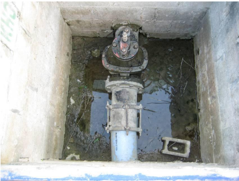
Figure 3-06: Sahanoa-Tabbara Storage Tank Outlet Valve
