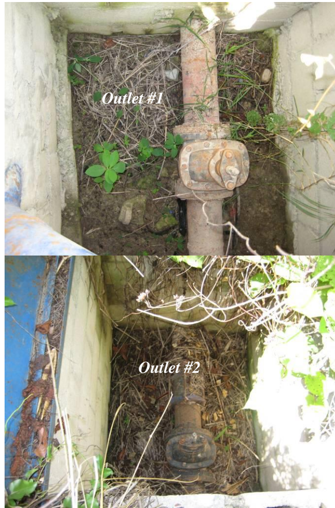
Figure 3-09: Chlorine Contact Tank Outlet Valves (out of service)
